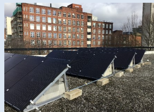
South-west array on roof of Ferranti building. Image: Nando Ochoa
